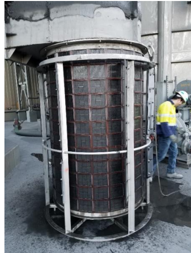
Figure 6. Derrick G-Vault™ Pulled from NGM Resin Circuit for Inspection (E. Mortensen)
